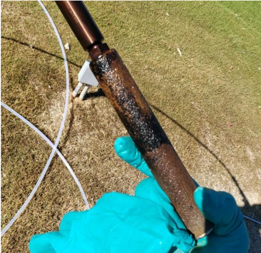
Before Diffuser Cleaning
